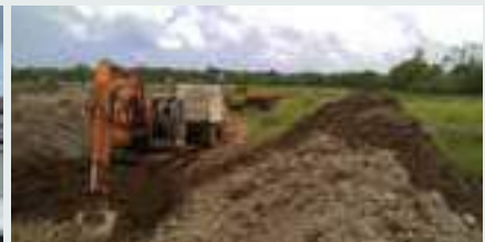
Assessment of clay mines of our suppliers to ensure the mines are adequately back-filled
