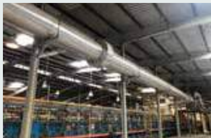
Ensuring safe emission of gases from the melting furnace and other energy saving initiatives
