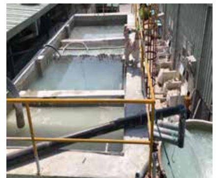
Squaring waste water treatment plant- Royal Caramics Lanka PLC_Horana Factory
