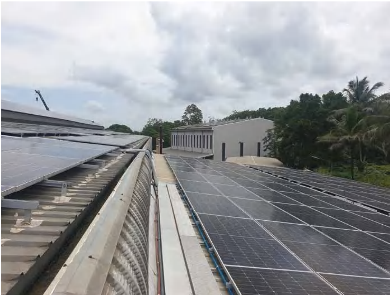
Renewable energy through solar power generation - Lanka Walltiles PLC-Meepe Factory
